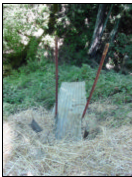
New culvert outlet drains into vegetation to dissipate drainage effect on slope.
